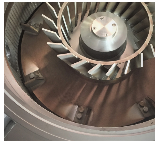
Detail of the grinding room
